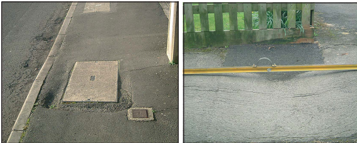
Depressions in footway (DEPR)
