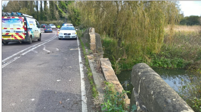
Structural damage (STRU)
