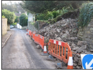
Structural failure (STRU)
