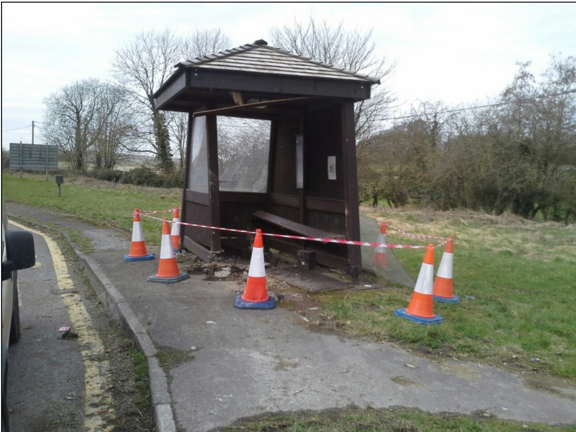
Street furniture structural damage (DAST)
