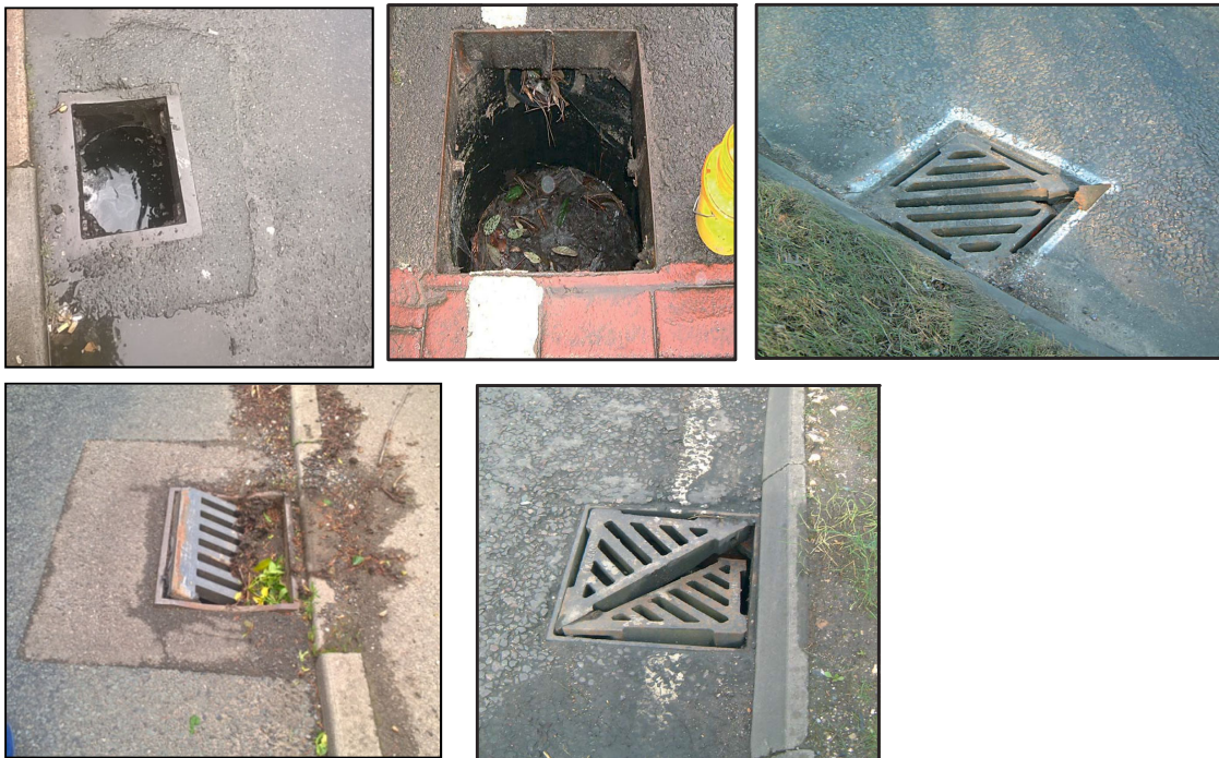
Cracked, missing, broken or level difference (IBCK, MISS, IDLV, LEVE)
