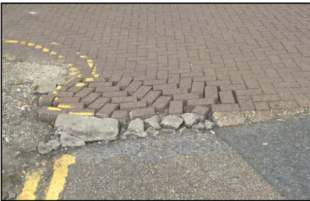
Footway trip, slab profile/rocking slab (SLPF)
