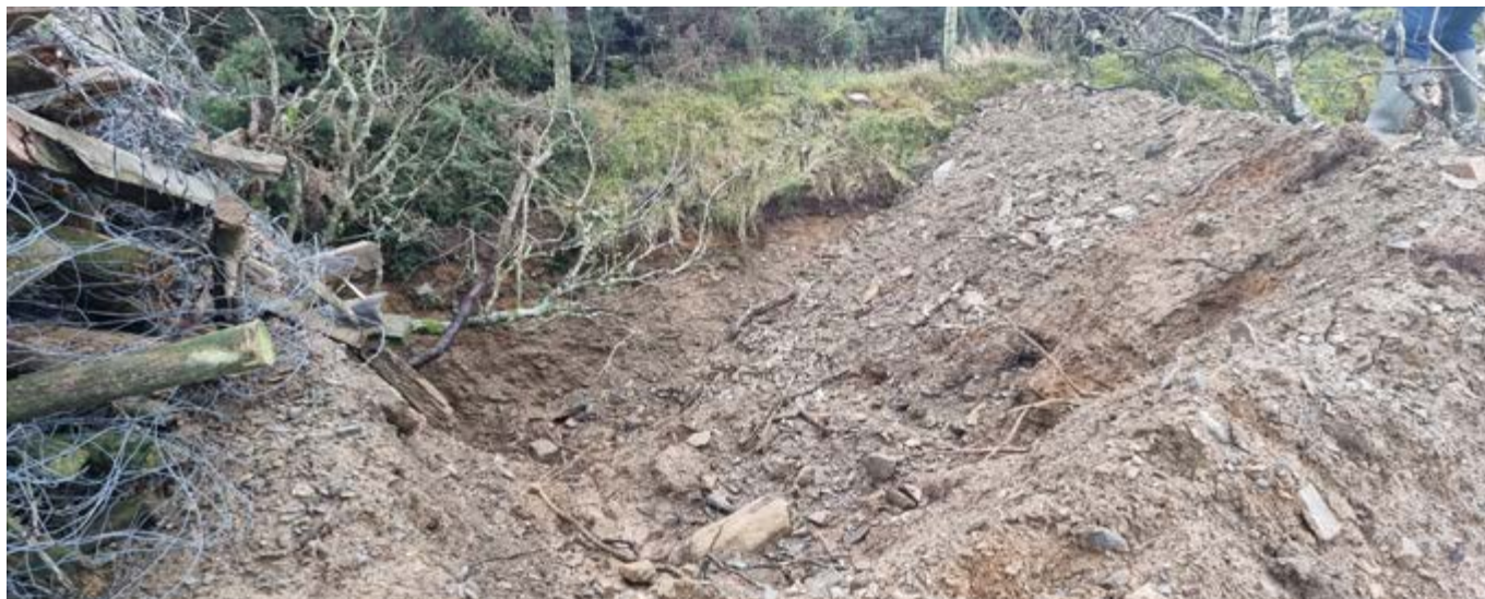
Photo: Excavation and obstruction of an unclassified road in North Wales to stop 'damaging' motorised use. The pit extends across the full width of the road and is more than 2m deep.
