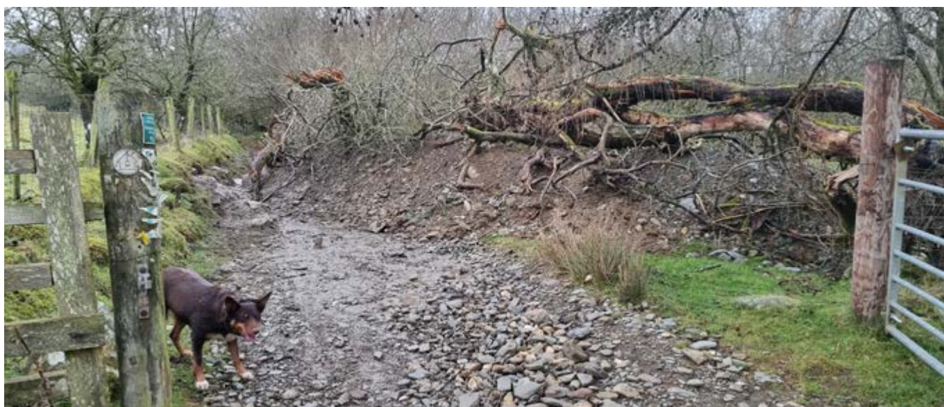
Photo: A green road excavated and blocked in several places to prevent motorised use because it is claimed to be 'damaging'. The material was dug out and behind it lies a large pit, this has filled with water diverted from an existing drain. This road lies adjacent to SSSI land and is unsafe for all users.
