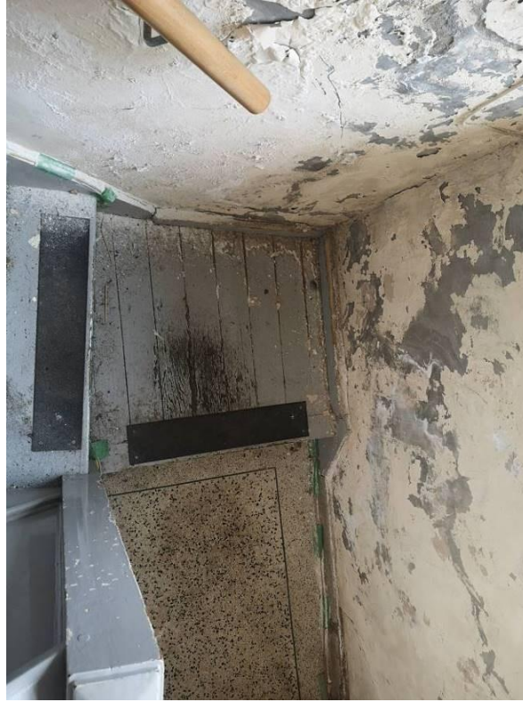
Photograph A2.11 – Serious damp penetration to internal stair walls.
