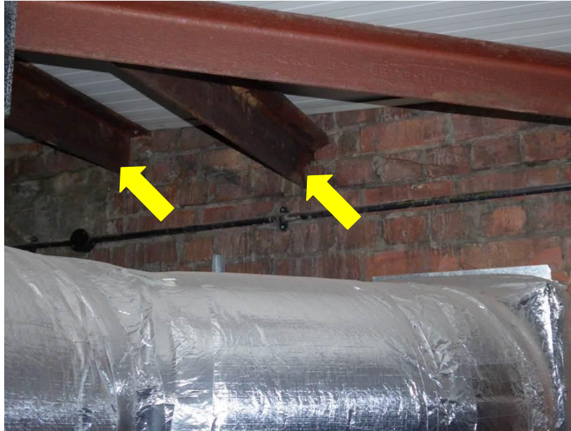
Photo 29 – Surface corrosion of purlins bearing on external wall.
