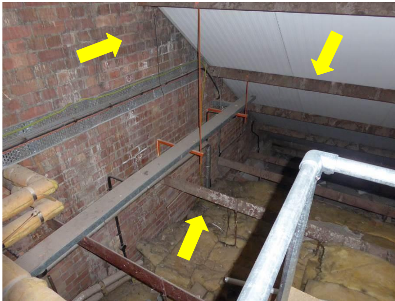
Photo 28 – Staining on supporting angles (secondary beams and purlins) and wall.
