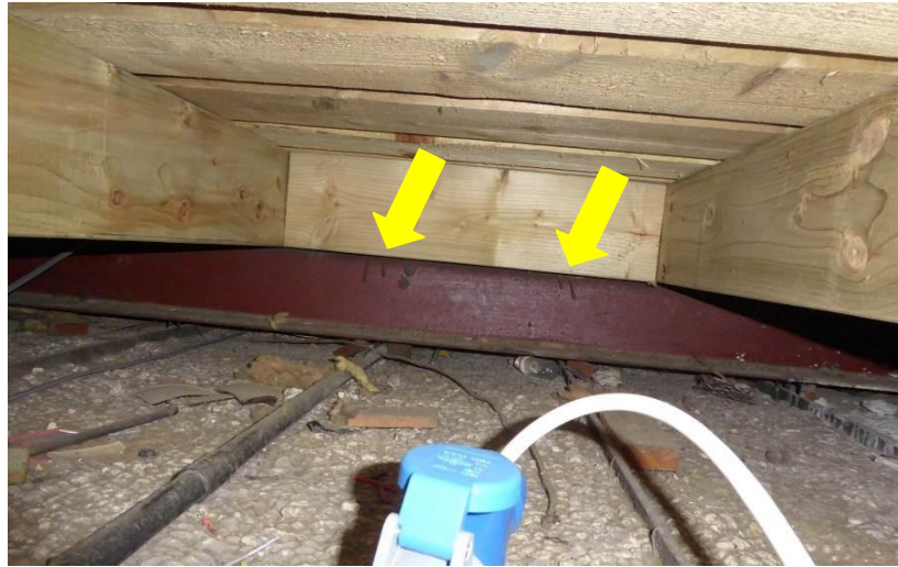
Photo 17 – Metal wire ties hooked over the angle arm.
