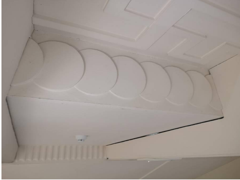
Photograph A3.5 – Typical gap between down stand lighting box and side lowered ceiling as shown in photo A3.2 above.
