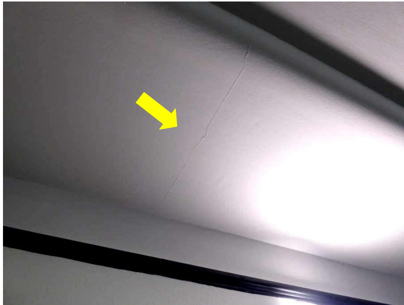
Photo 7 – Crack in Foyer ceiling.
