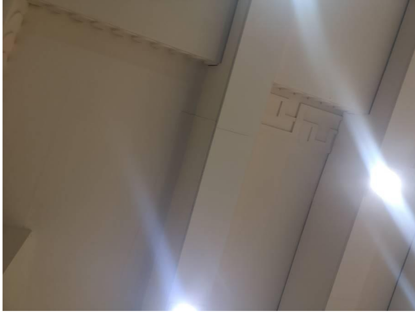
Photograph A2.1 – Auditorium ceiling showing downstand lighting boxes and section where there is no Greek key between High level and lowered ceiling. Possible recent repair.
