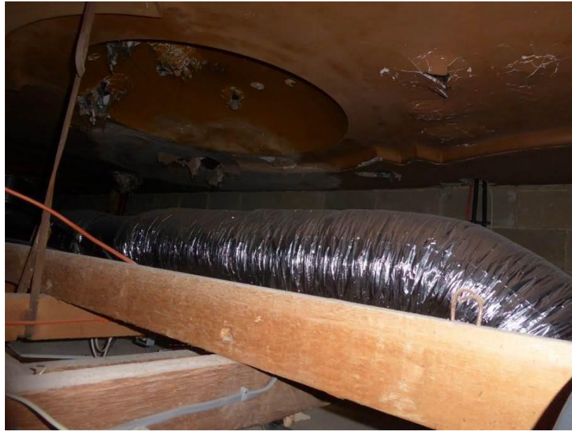
Photo 35 – Damaged underside of the ceiling over the Alamein Room.
