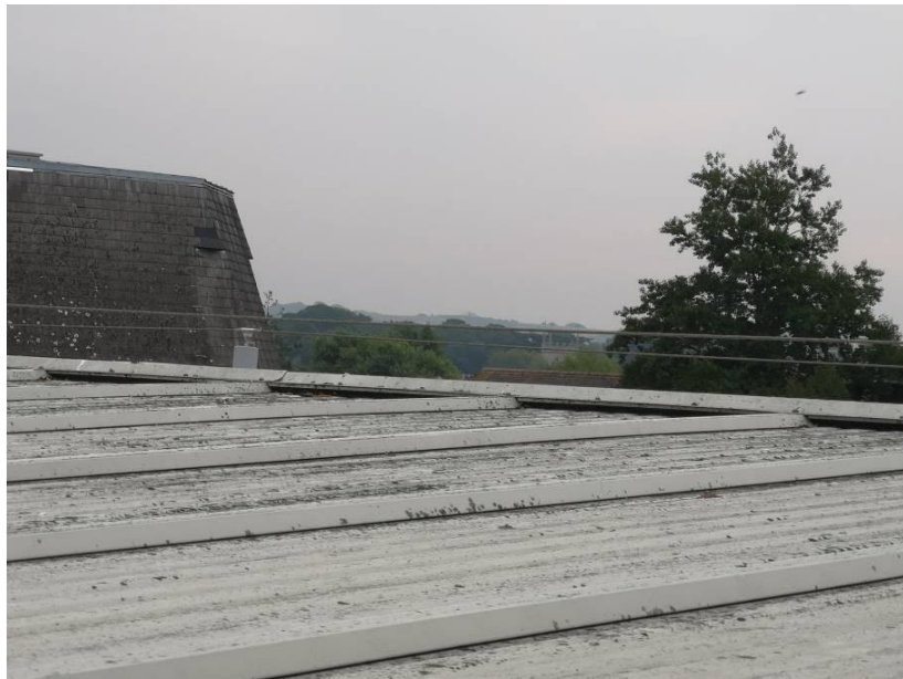
Photograph A2.4 – Looking across roof towards the east – note east ridge line flashing is in place.
