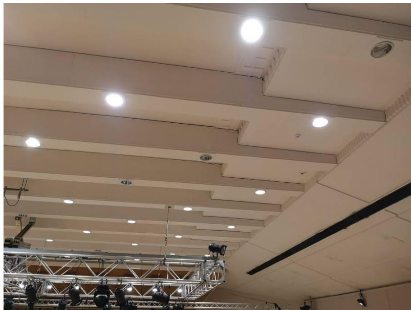
Photograph A3.2– Main auditorium ceiling on third visit showing vaulted ceiling to the side.
