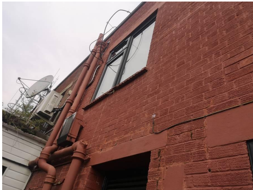
Photograph A2.12 – Part east elevation – Note brickwork has been painted with a non-breathable paint.
