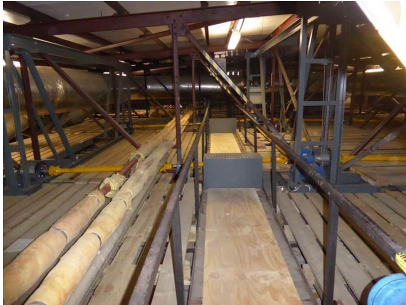
Photo 12 – Services in loft above Auditorium.
