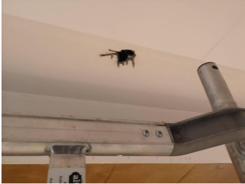
Photograph A3.7 – Hole noted to side of light fitting near to stage – appeared to have 'burnt through'
