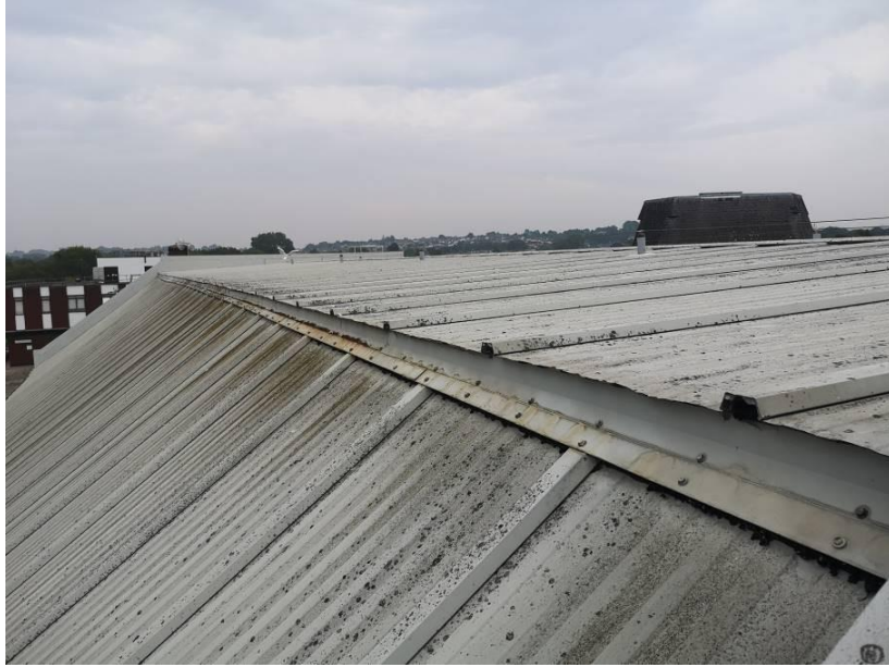
Photograph A2.3 – West elevation, look north along ridge line to main auditorium roof – note the missing ridge flashing.
