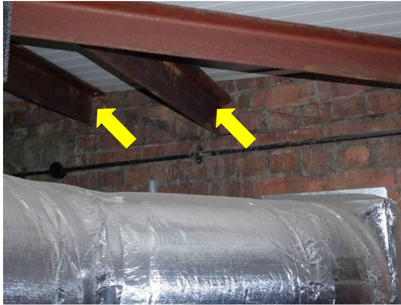
Photo 31 – Surface corrosion of purlins bearing on external wall.
