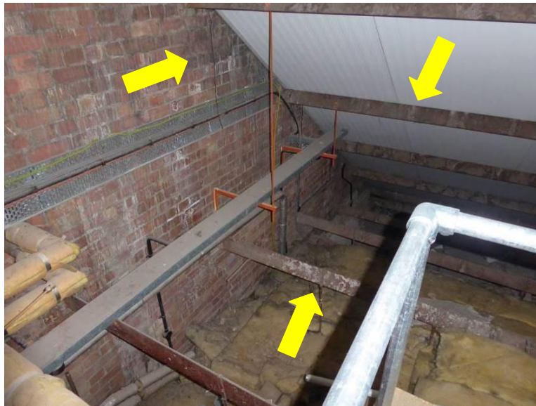
Photo 30 – Staining on supporting angles (secondary beams and purlins) and wall.
