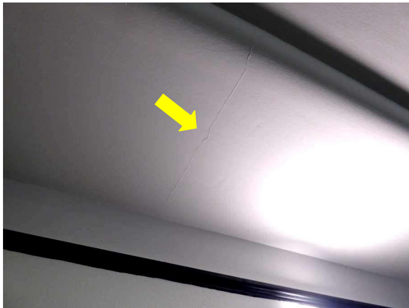
Photo 7 – Crack in Foyer ceiling.
