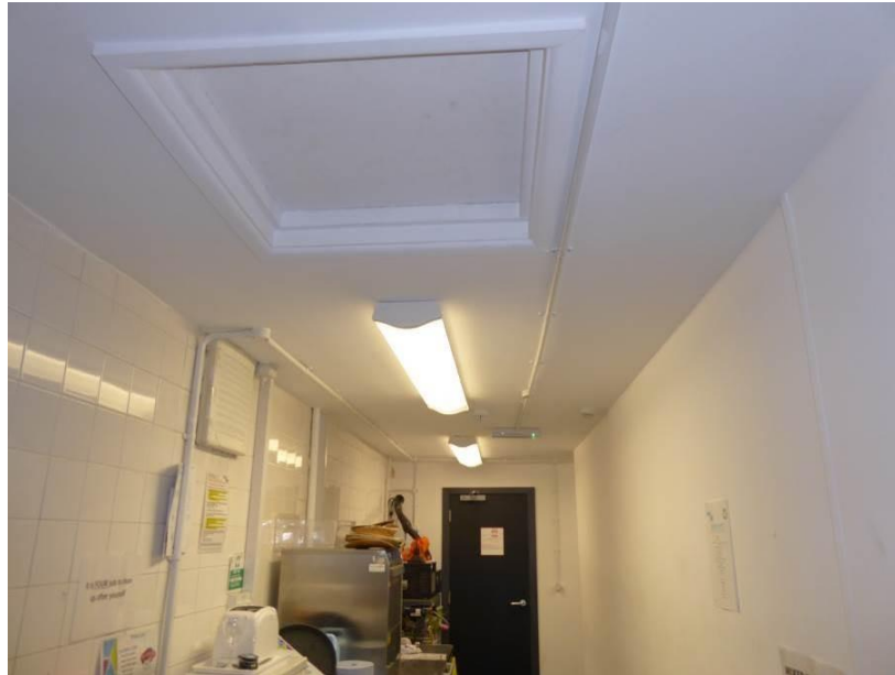
Photo 9 – Ceilings over the Kitchen.
