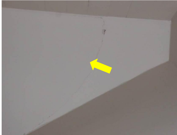
Photo 24 – Crack to the left-hand side of the stage.
