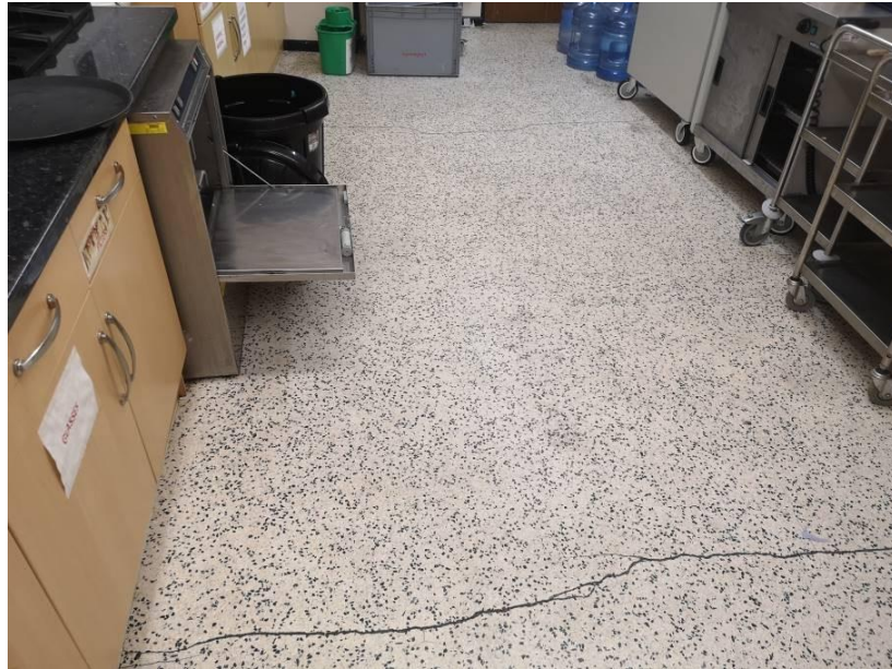
Photograph A2.13 – Regular east/west floor cracks to kitchen terrazzo finished floor at first floor level.
