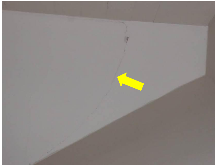
Photo 26 – Crack to the left-hand side of the stage.
