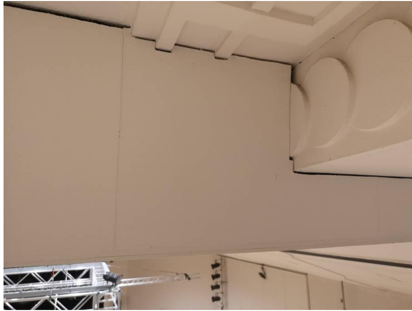
Photograph A3.3 – Typical detail of downstand lighting box showing gaps between horizontal and vertical boards.
