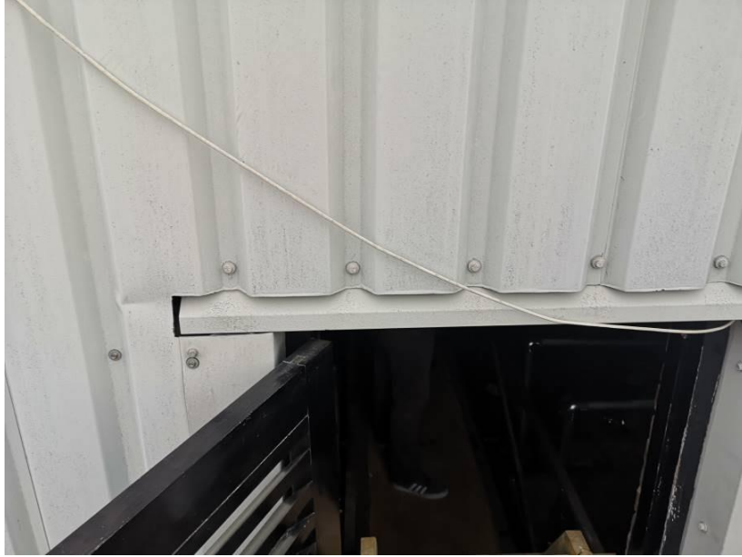
Photograph A2.5 – South elevation roof access door - Note the poor fitting flashing to top of door.
