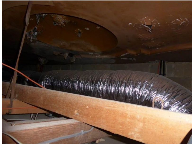
Photo 32 – Damaged underside of the ceiling over the Alamein Room.
