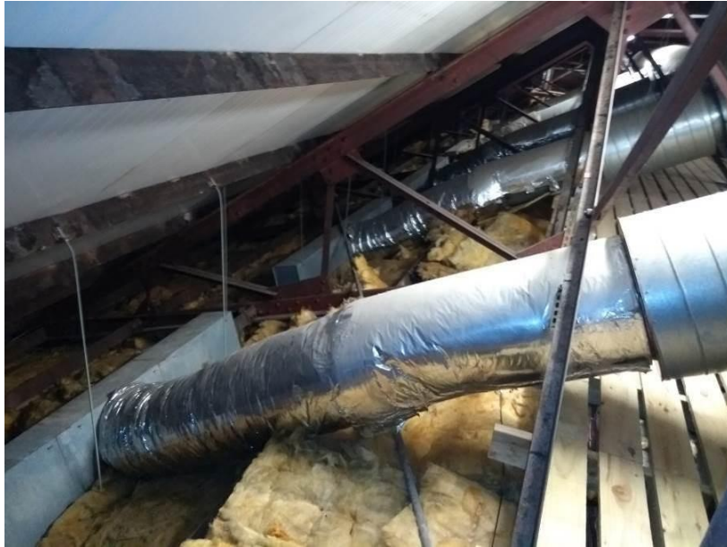
Photo 15 – Loft over vaulted ceiling -vent ducts, no timber decking for access.
