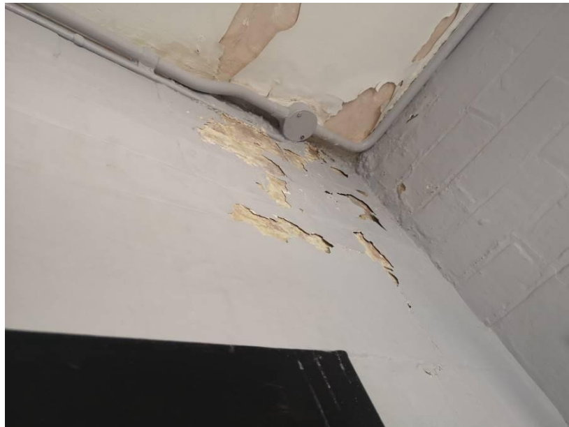
Photograph A2.16 – The dressing rooms to the north-east corner exhibited signs of severe damp penetration.
