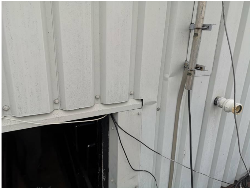
Photograph A2.6 – South elevation roof access door - Note the poor fitting flashing to top of door.
