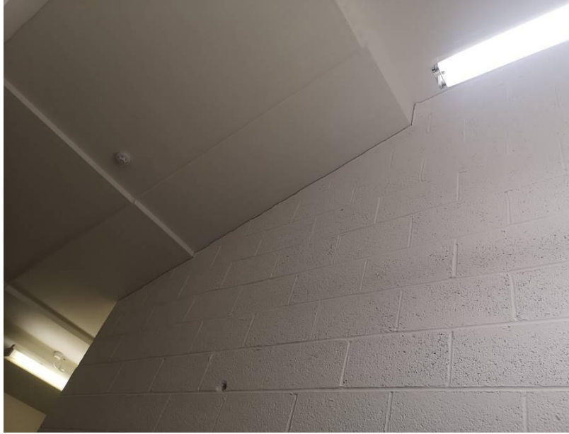
Photograph A2.9 – Gap at top of recently painted wall to SpireFM offices.
