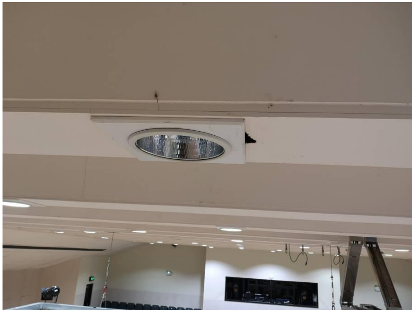
Photograph A3.6 – Typical light fitting to bottom of downstand showing over-sized opening in plasterboard.
