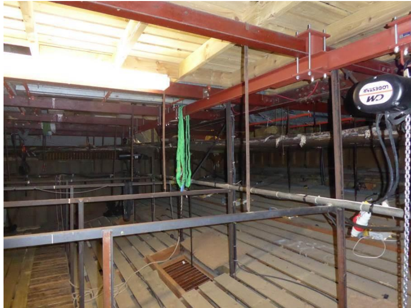
Photo 22 – Steel subframe supporting lighting rig.
