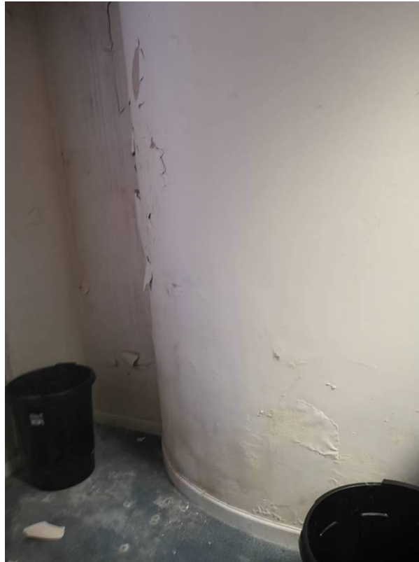
Photograph A2.15 – Curved wall to abandoned ground floor offices showing serious signs of damp penetration.
