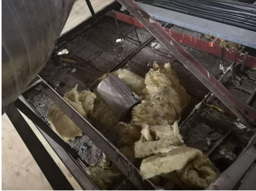
Photograph A2.7 – Loft side of high-level roof – showing numerous openings.
