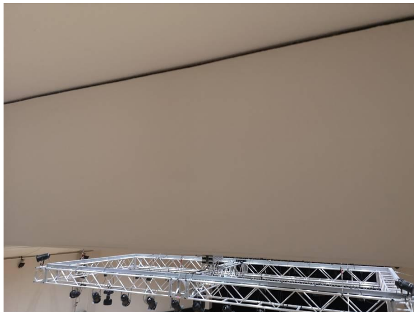
Photograph A3.4 – Typical gap between down stand lighting box and main ceiling as shown in photo A3.3 above.
