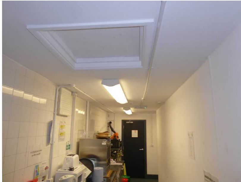
Photograph A1.9 – Kitchen ceiling.
